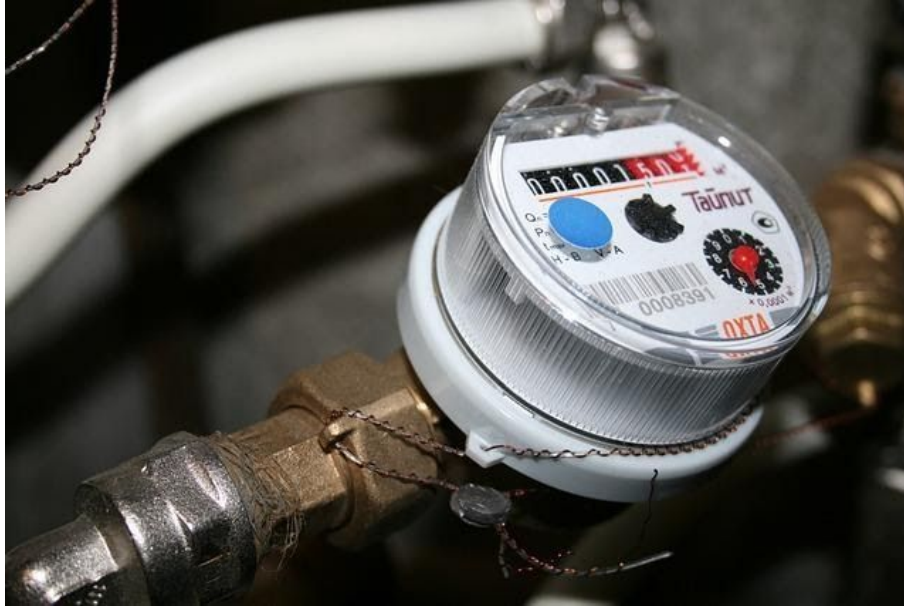
Water meter reading
