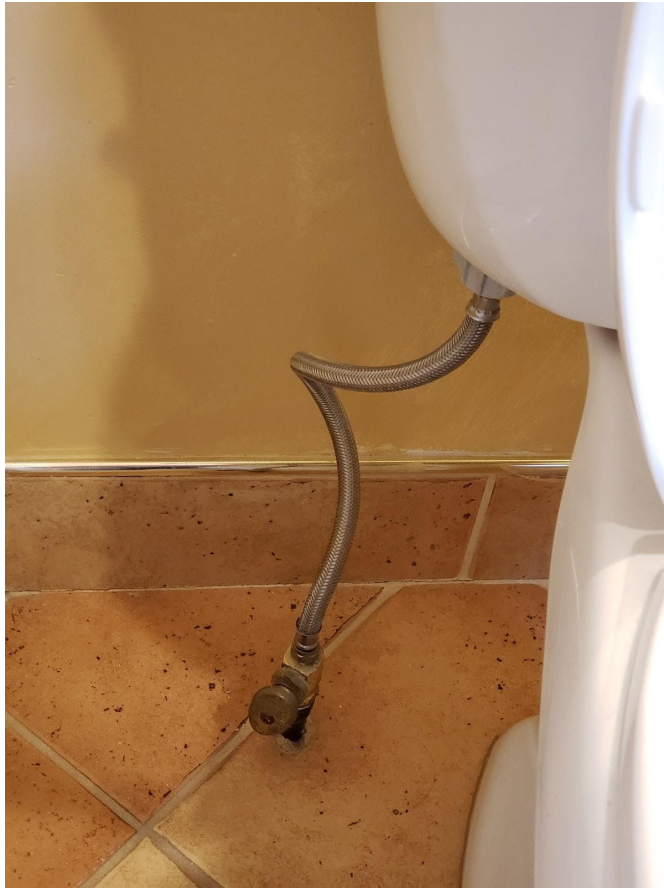
Toilet stop valve
