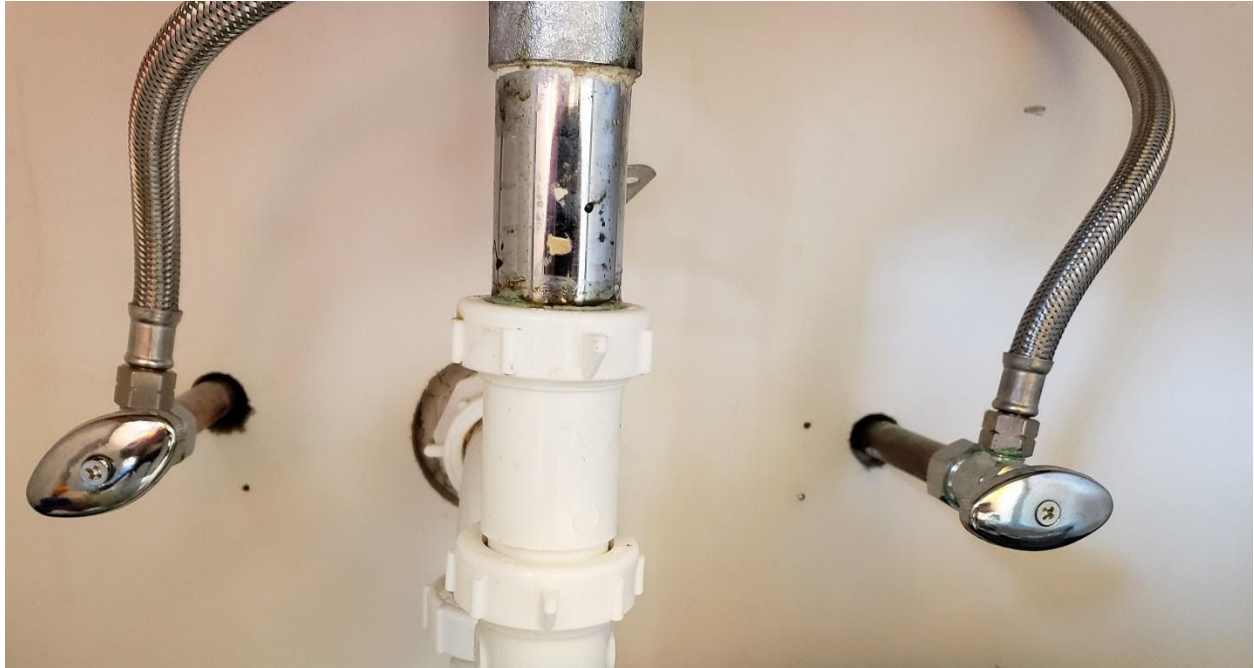
Bathroom sink chrome-plated stop valves
